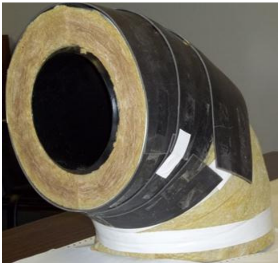
Figure 7 – Mass loaded vinyl mitered sections (gores) placed around insulation with longitudinal joint at about 3 o'clock and with required \geq 1.3 cm ( \geq \frac{1}{2} inch) longitudinal overlap. Also shown is overlap at circumferential joint which is required to be a maximum of 1.3 cm ( \frac{1}{2} inch).
